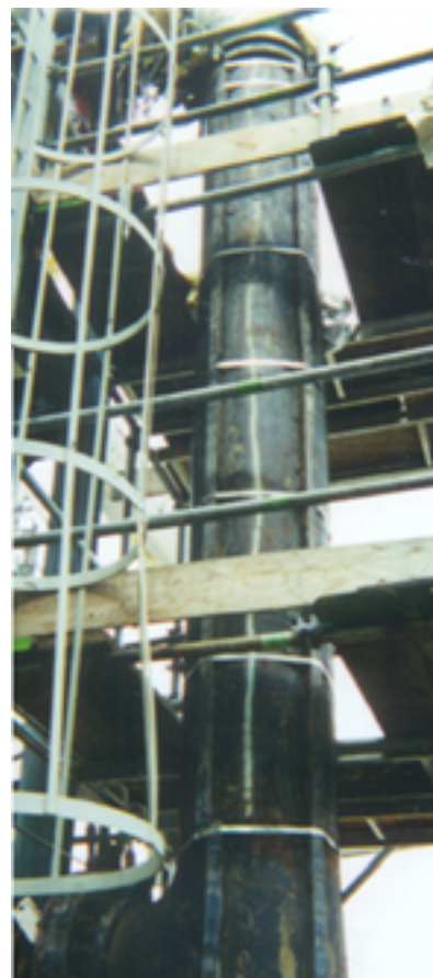
The sulfur pipeline at an Alberta, Canada, Canada, The natural gas plant has been operational for one and a half years since installation
