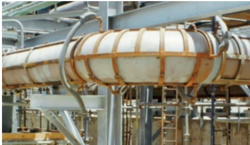
Fig. 2: Approximately four miles of Controls Southeast ControTrace® type bolt-on jacketing has been installed on this terminal’s main sulphur transfer line.
