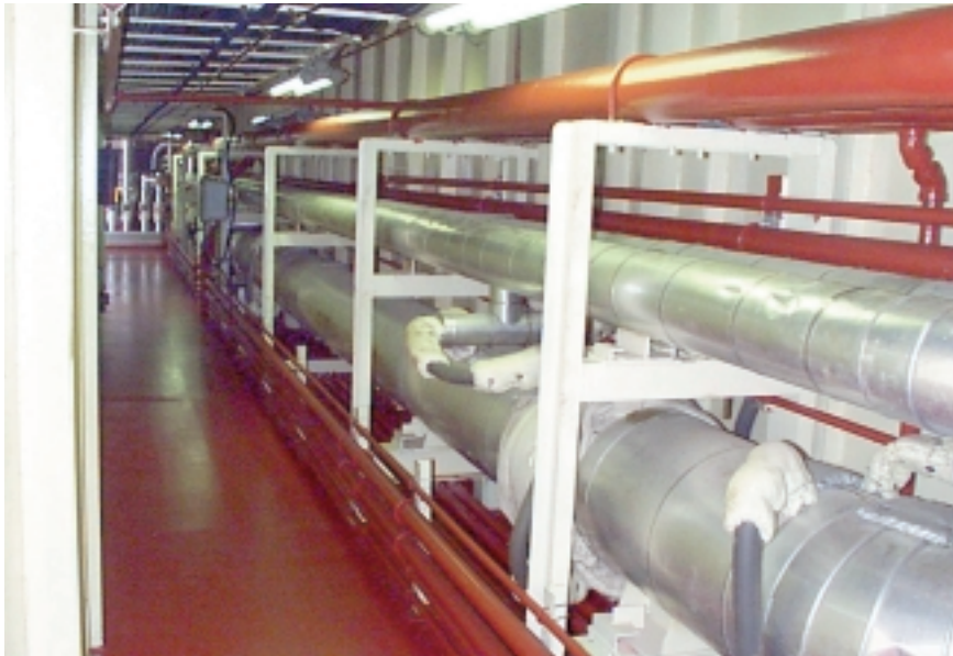
Fig. 4: Bolt-on thermal maintenance systems have operated trouble-free on the Sulphur Enterprise since the ship's launch in 1994.
