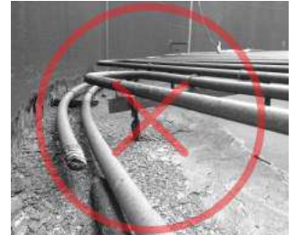
Failed Internal Coil
