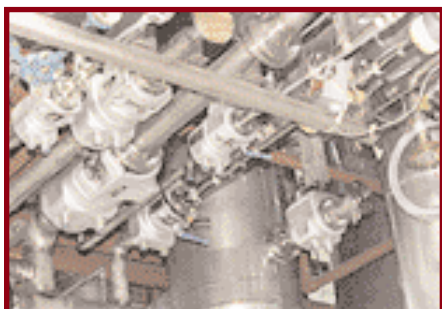
Hundreds of bolt-on jackets were used for temperature maintenance on the valves in this jacketed system.
