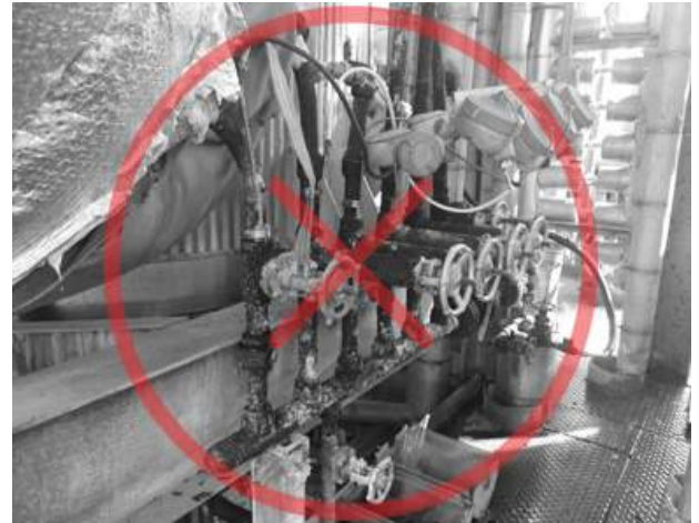
Forgotten Plant Infrastructure: The lines shown above tie into one steam trap, which results in condensate back-up and poor tracing performance.
