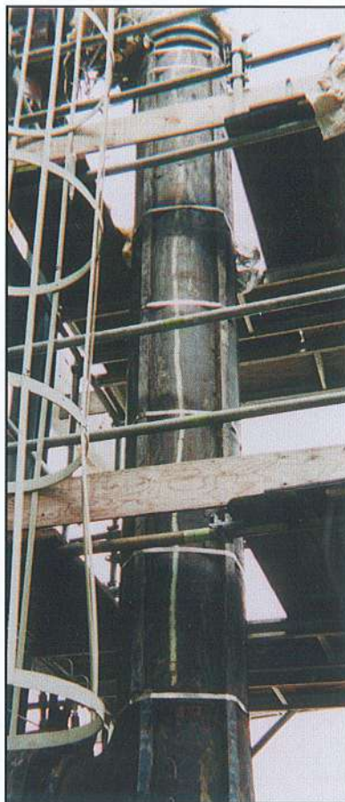
The sulfur pipeline at an Alberta, Canada, natural gas plant has been operational for one and a half years since installation of new bolt-on heat trace elements.
