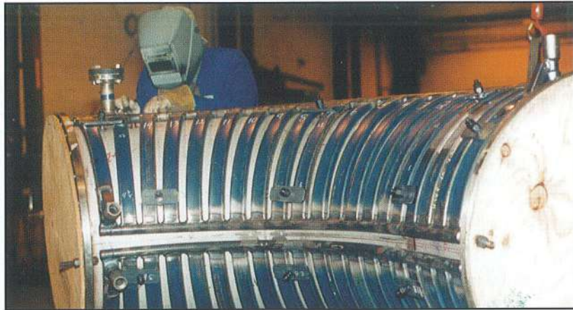
To help prevent plating in the waste gas header, a producer of a common anhydrous material installed new bolt-on heat trace elements to keep the header's wall at a uniform temperature.
