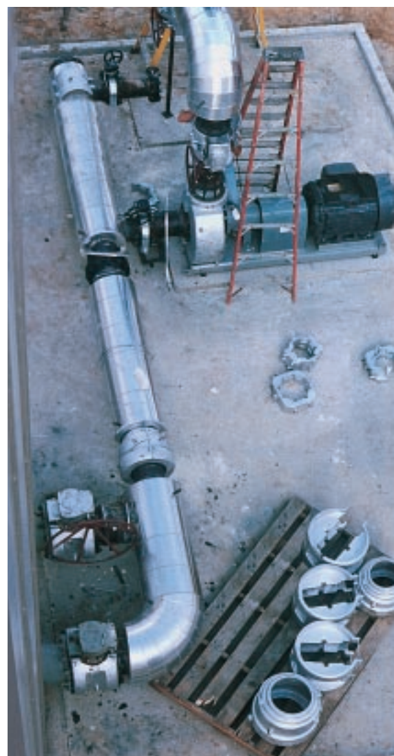
At Martin Gas' new Beaumont facility, ControHeat bolt-on jackets, like the ones pictured on the Flowserve Mark III centrifugal pump, the 12 inch Tufline butterfly and plug valves adjacent to the sulphur storage tank, and the Hyspan ball joints will be used to maintain temperature on all the process equipment. All of the 6 in., 10 in. and 12 in. transfer lines will be heated with a ControTrace thermal maintenance system.
