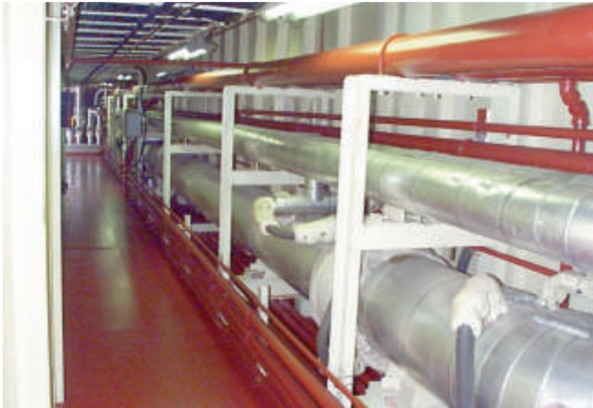
Fig. 4: Bolt-on thermal maintenance systems have operated trouble-free on the Sulphur Enterprise since the ship's launch in 1994.
