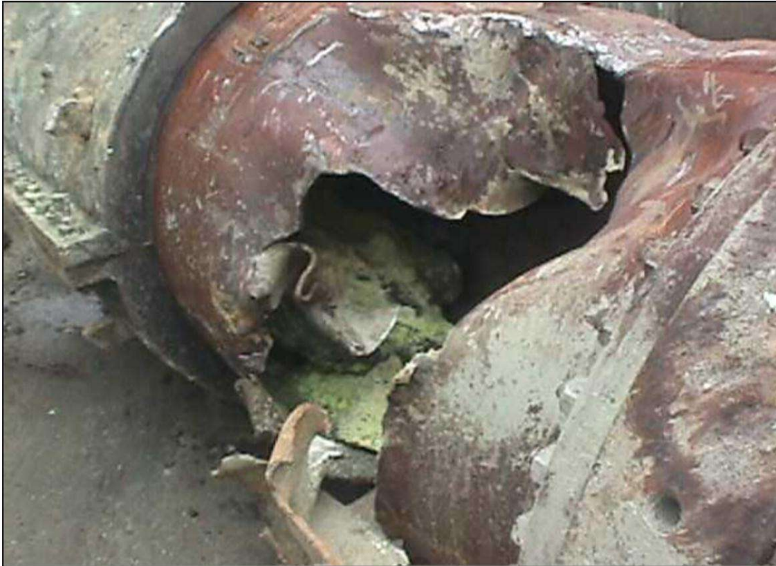
Figure 3: SRU Vapor Line Failure due to Extreme Corrosion
