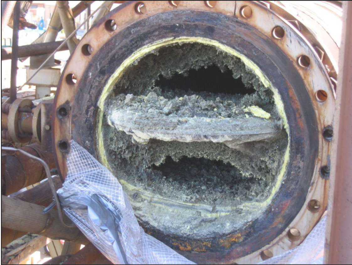
Figure 4: SRU Vapor Line Failure due to Plugging
