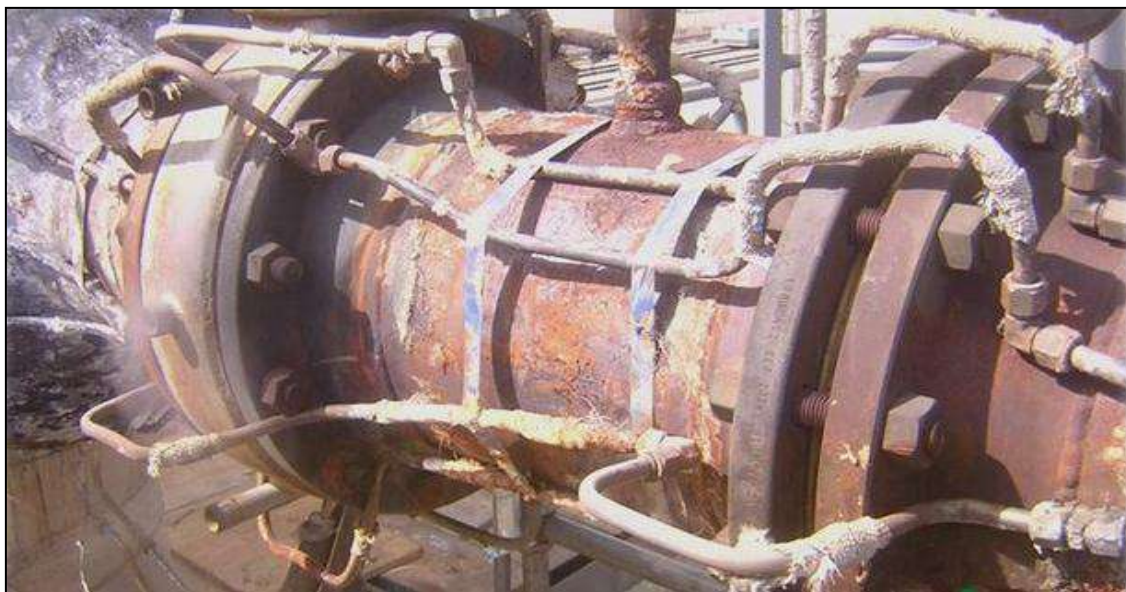
Figure 2: Convective Tube Tracing Installed on Large-Bore Piping
