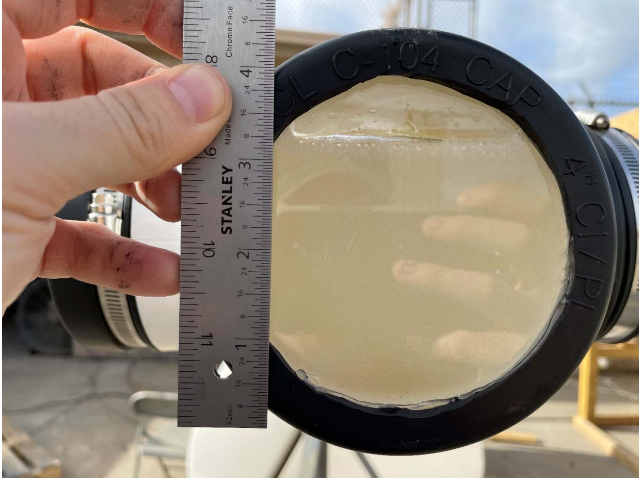
Example of liquid level viewed through sight glass on horizontal rod-out elbow
