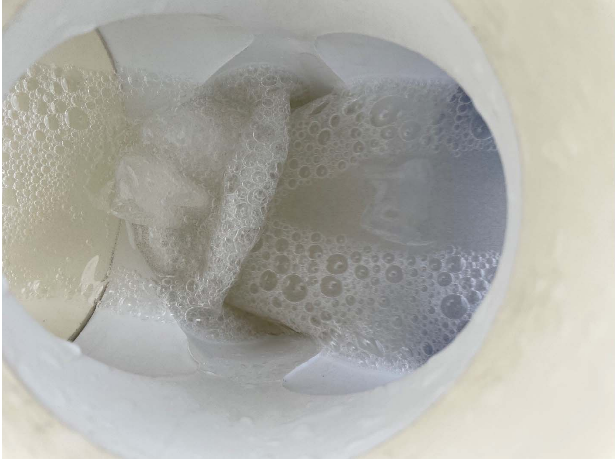
Example of liquid flow through the vertical drop; view from above
